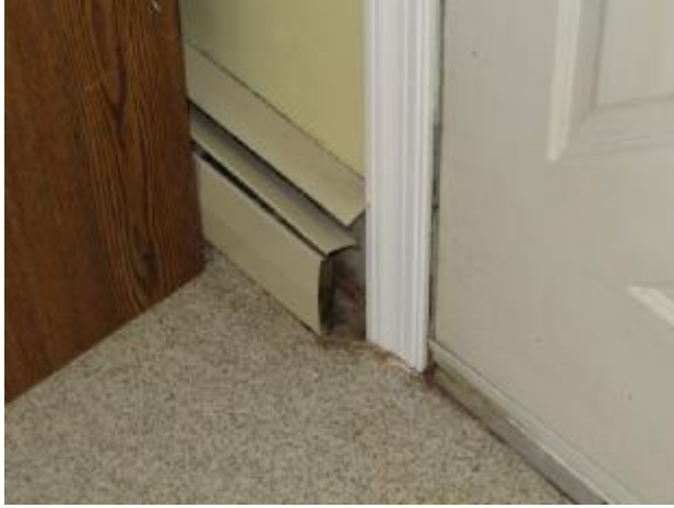
Missing end cover
