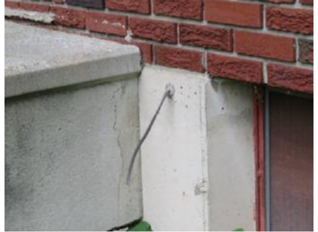
Incomplete electrical circuit
