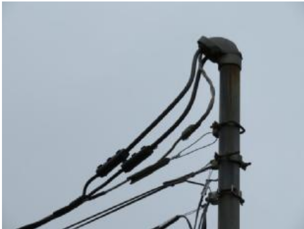
Inadequate drip loop
