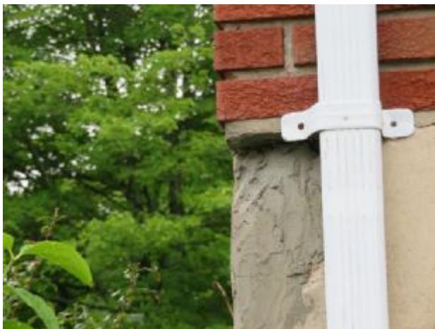
Broken foundation corner
