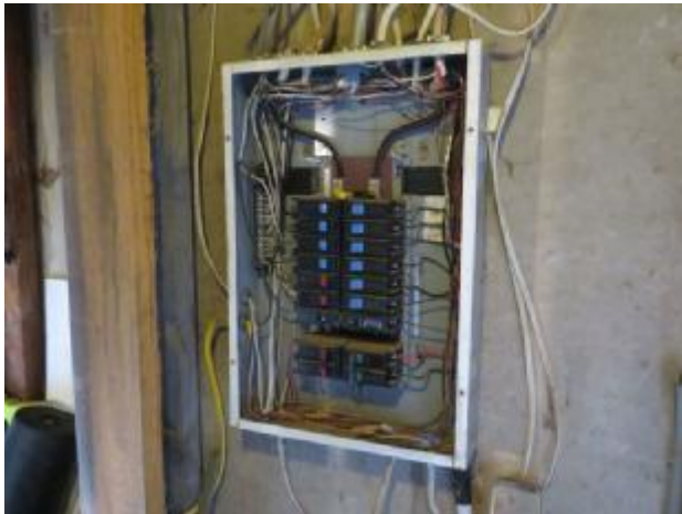
No main breaker
