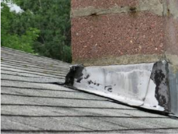
Loose flashing and no cricket
