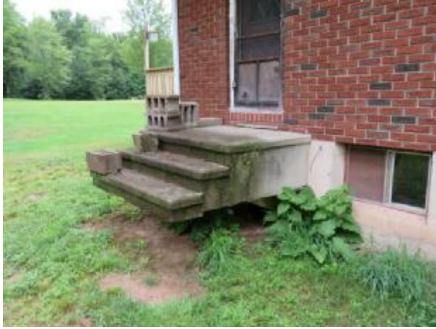
Incorrect stairs with no railing
