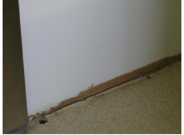
Missing base trim
