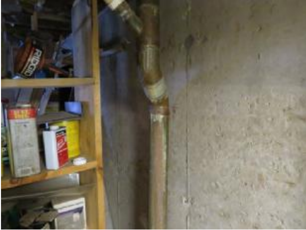
Incorrect repair on waste pipe
