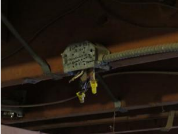
Uncovered junction box.
